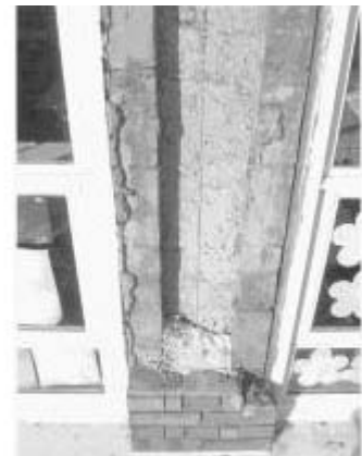
Concrete casing with no ties to brickwork cladding
