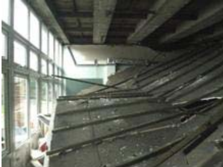
Ceiling and heaters after collapse
