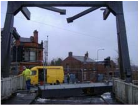
After failure with counterweight across carriageway
